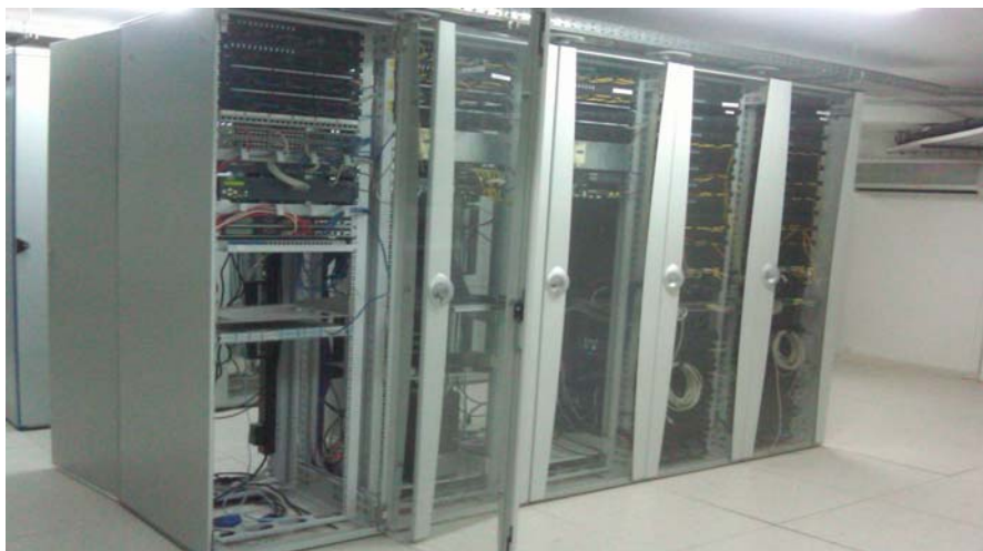
Figure II.4 - Fibre optic exchange located within the Industrial Consortium of Sulmona
